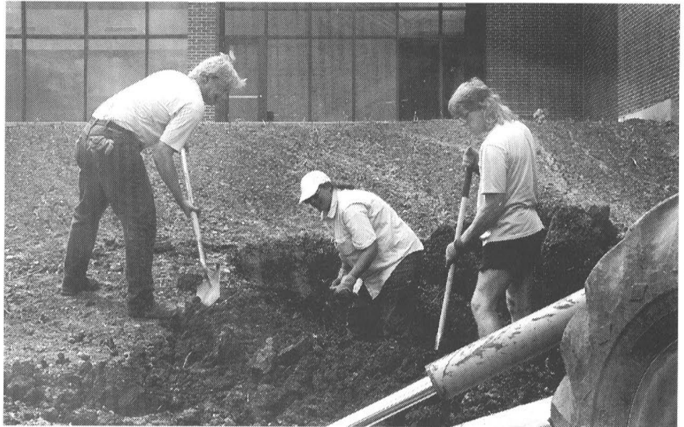
Harper's intern supervisor Tim Lembke, left, works with students Marla Daly and David Kraft to alleviate drainage problems outside of Building L.
