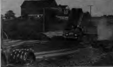
Euclid Ave. is paved, but this construction on Roselle Rd. will take more time. (Photo by John Kern)
