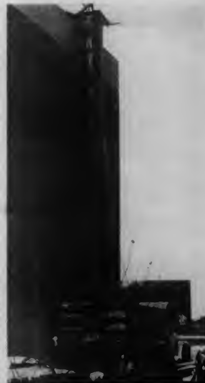
Repairs to the roof on Bldg. A have been slowed down by the snow. Unexpected weather conditions have put the repair project behind schedule.
