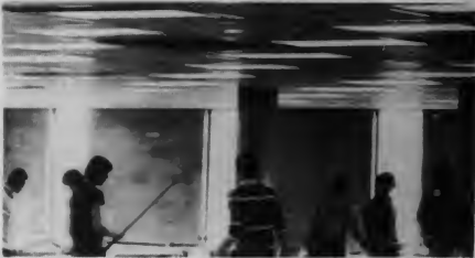
THE SKY IS falling, the sky is falling. Snow-laden roofs sprang leaks in the aftermath of the record snowfalls and rolling tiles, soaked with water, have been taken down in numerous areas on campus. Maintenance personnel have been kept busy with mop-up operations and the leaks are expected to continue through the day. (Photo by Steve Mackay)
