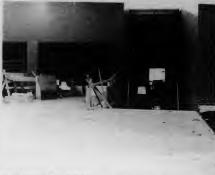
The entrance to Bldg. M is nearly finished. Some of the athletic site swimming pool. The building to inspect the facilities provided by the building will be tennis, and to be done in early spring. (photo by Mike Wendes)
