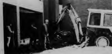
Construction men work to repair the broken water main behind D Bldg. Harper was without water for several days, but water was probably restored in most of the buildings by early last week. (photo by Scott Aronson)
