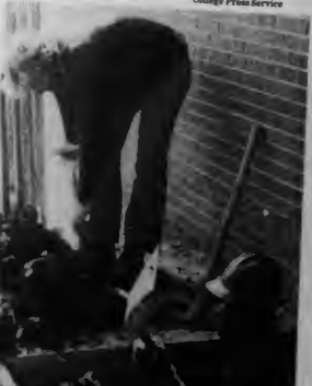
The repairs being made on A 1044, continue. As this worker is up to his shoulders in dirt, the other men engage the gravel from the pavement behind him.
