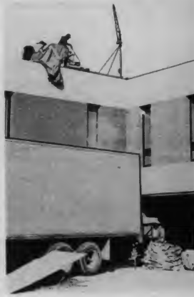
Building repairs changed campus, and stank up the air. Repairs were completed Monday. (photo by Rick Kibick)
