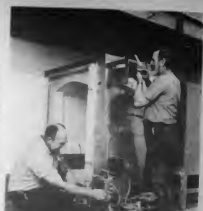
MAINTENANCE PERSONNEL put the finishing touches on the new gas kilns installed in Bldg V. The building was redesigned to accommodate sculpture, ceramics and three-dimensional design facilities. (Photo courtesy of Harper College.)
