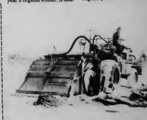
Construction began late last week for widening the perimeter road in the back of the campus. Photo by Bob Reed.
