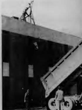
According to Don Masic, director, physical plant, roof repairs will be completed by the end of the year. Photo by Paul Proccocio.
