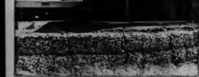
Construction is well underway as the new warehouse reaches completion. Once completed the warehouse will store a wide variety of campus supplies. Space for the warehouse, which will be the college's first, is being provided by expanding Building B. Photo by Bob Falk.
