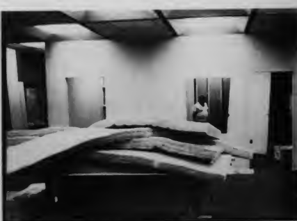
Workers are busy finishing up the new rooms in the Harper library. These rooms will house the Kurzweil reader and the enlarged reader for disabled students. Photo by Bob Nank
