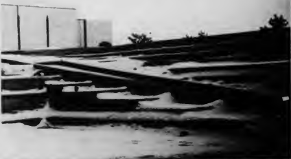
The south patio, under construction in front of Building A, will offer an alternative eating environment upon completion, with trees, flowers and other assorted floral. Spring fauna watching should be a premium attraction to many wildlife enthusiasts.
