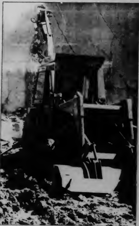
A lone bulldozer stands guard over the college campus during major reconstruction work in front of Building A.
