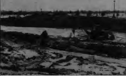
The lot south of F Bldg undergoes major foundation work. Several entrances to the bldg are temporarily closed. (Photo Credit - Cheryl La Croix)
