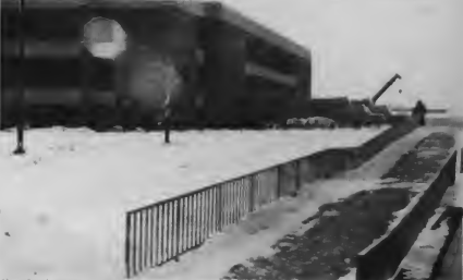
Completed projects include this ramp near C Bldg and some sidewalk resurfacing. Still awaiting completion are the stairs to F Bldg library and the restructuring of the retaining walls between F Bldg and A Bldg.
