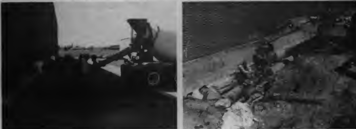
Construction continues as workers pour concrete and lay drainage pipe in an effort to improve the look and safety of Harper's campus. (Photos by Tracy Brown)
