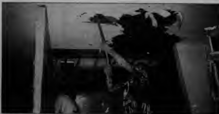
Two members from the demolition crew tear down the ceiling in building I during the construction project that lasts until the fall.
