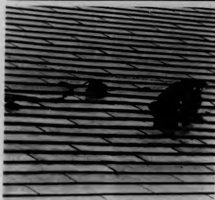
A solitary workman fixes leaky roof over lecture hall E-106. (Photo by Tom Newhouse)
