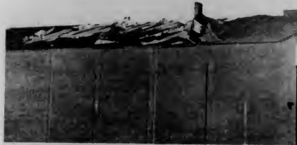
Plastic strips, sheeting, and insulation are ripped from the roof of "P" building. (Harper staff photo)
